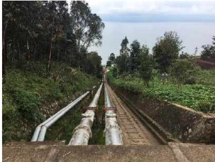
Figure 20: View of the penstocks supplying the Gisenyi hydropower station.
