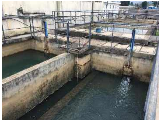
Figure 17: Gihira Water Treatment Plant in Rwanda (October 2020)
